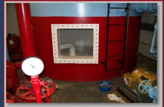
MCCRORY INSTALLED MAN WAY
