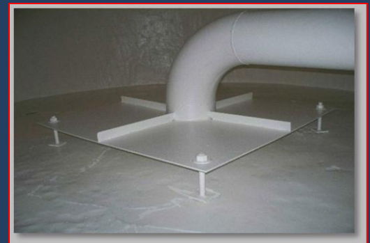
MCCRORY INSTALLED ANTI-VORTEX PLATE
